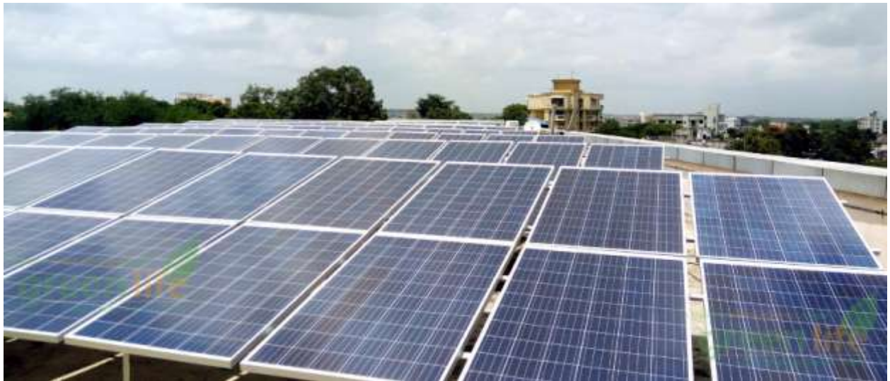
Solar Plant installed at College Premises
